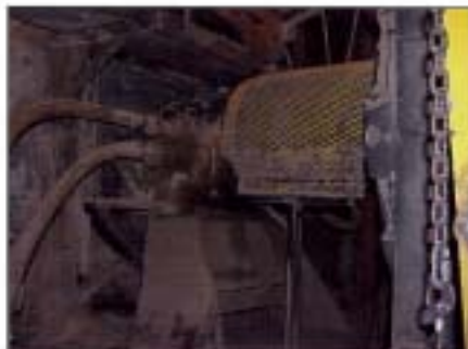
Another view of the balancing system installed on the E24 fan.
