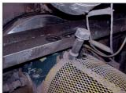
Close-up view of the balancer installed on the E24 fan. The top portion of the balancing ring is visible.
