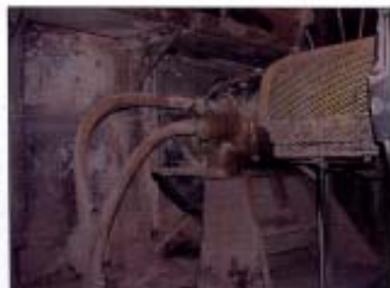
Lord fan balancing system installed on Buffalo Forge (Howden) E24 Preheater fan. The fan is 104 in. dia., 1200 Hp and runs at 1180 rpm.
