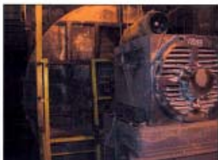
Lord fan balancing system installed on Buffalo Forge (Howden) 57.5 in. dia., 75 Hp, 1800 rpm ID Fan.
