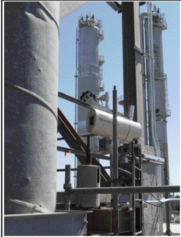
The 14 Mikron IR cameras are located at distances of 10 to 40 ft. from the gas separation unit. Real-time radiometric temperature data is transmitted by wireless Ethernet from each camera to a control room 1100 ft. away
