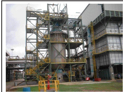
The largest radiometric imaging system for safety monitoring of a petrochemical processing vessel uses 14 Mikron IR cameras and MikroSpec™ R/T Software. It has been on line for over two years monitoring this Chevron-Texaco-designed gas separation system in Texas.
