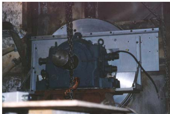
Figure 6. Installation at GCC Dacotah Cement
