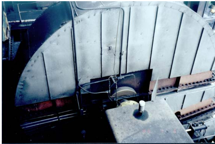
Figure 7. Installation at US Steel, Gary Works
